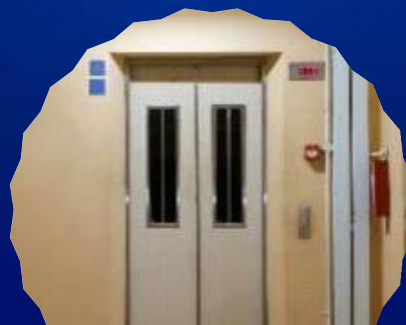
Fire Evacuation Elevator
